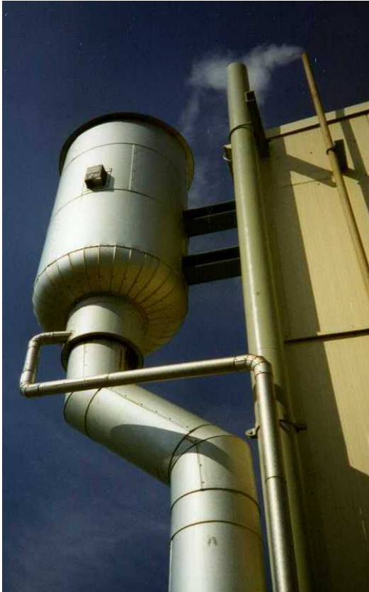
Vent silencer at Piesteritz Plant
