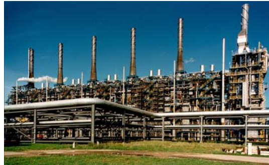
Multiple vent silencers at a single process section
